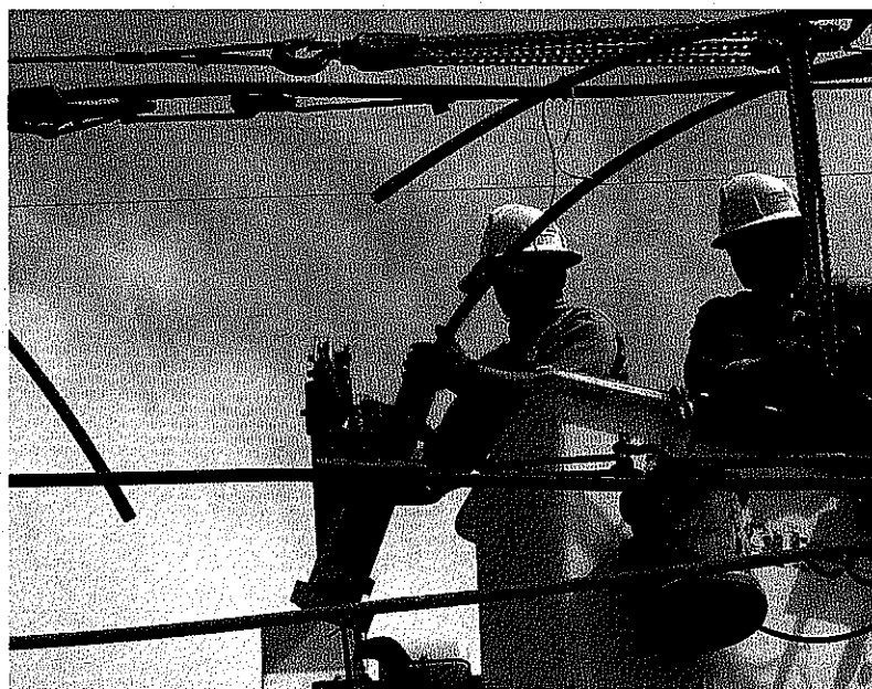
Southern Company became one of seven utilities to participate in a research project to solve an ongoing problem with conductor failures.
